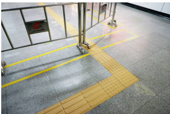
图3 被铁马护栏阻断的盲道 Fig.3 Blind tracks blocked by guardrails
