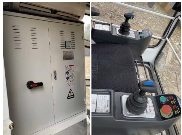
图4 塔机驾驶室电源箱和操控台 Fig.4 Power box and control console of tower crane cab
